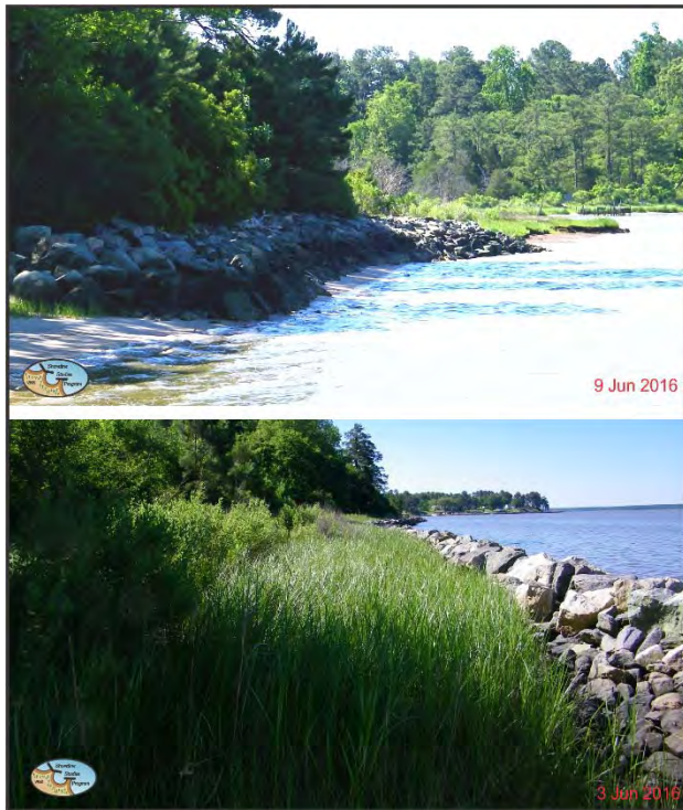
Figure 7. Top: Existing revetment along Werowocomoco. Bottom: Existing continuous high sill along the site.
